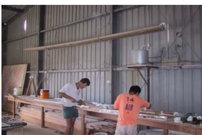
Building the catwalk, note beam hanging on wall. Small items can be built early.
