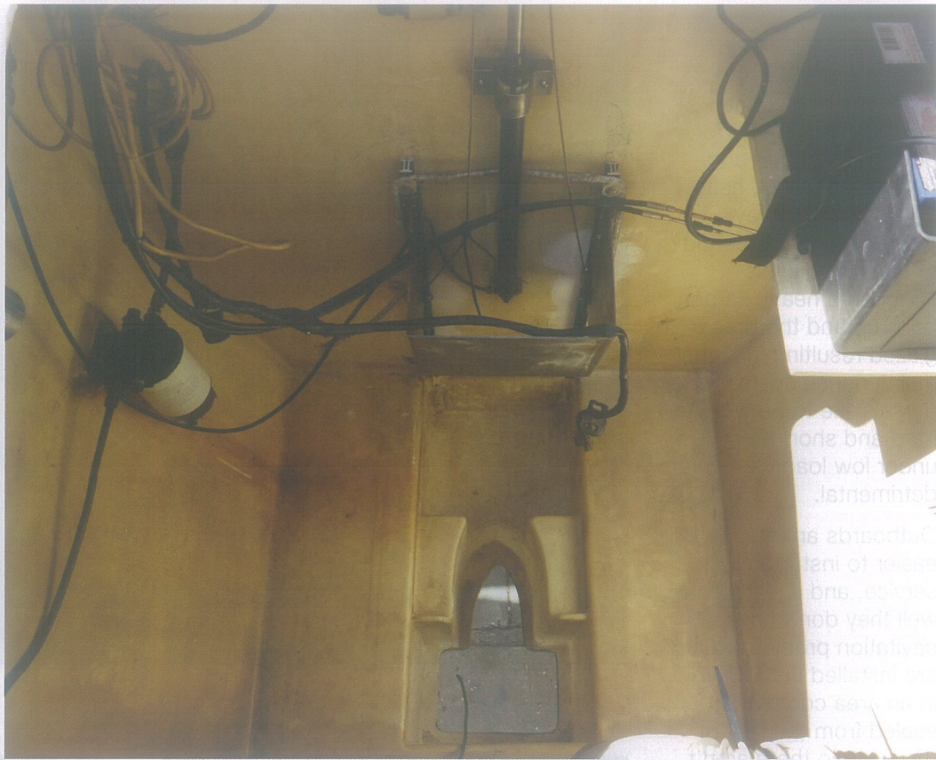
Motor removed for service.
