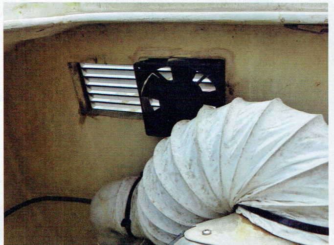
Fan extracts warm air from the top of the motor bay. Ducting goes to motor cowl for fresh air intake.
